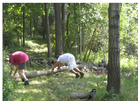
Paul and Jeremy Beech working on Beaver Log Wall at Pipestave last fall
